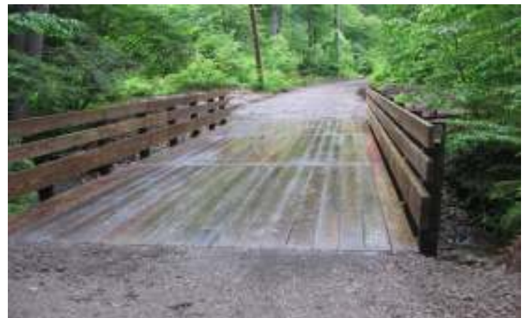
This picture is the finished Straight Run Bridge, located a half north of Duhring on ANF Snowmobile Trail 1
