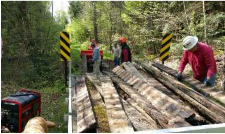
Jerry Thornton, Dan Stevenson, Hank Bauer, Dave Timothy and Jerry Beichner tear out and haul old timbers away from Straight Run Bridge
